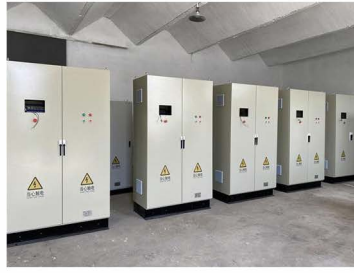
Energy storage system
