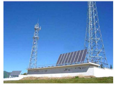
Communication base station, etc.
